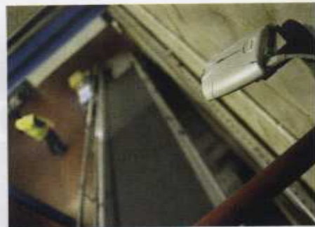
Cameras in the loading bay area have to be able to cope with extreme temperature fluctuations during winter.
